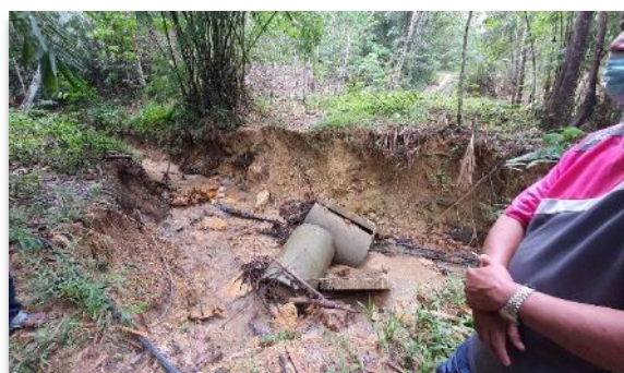
Figure 1 – Site of the collapse bridge.
